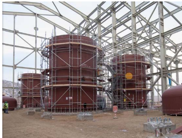
Flash vessel assembly on site
