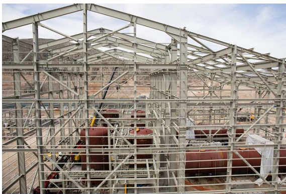
Autoclaves & Flash Vessels in POX Building
