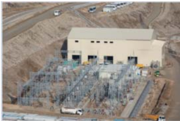
High Voltage Switchyard
